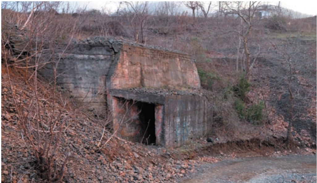
Fig. 76. Entrance of a small concrete bunker at Arrëz above the Miraka bridge (Elbasan Pref.); a hibernaculum of Rhinolophus ferrumequinum and Hypsugo savii . Photo by M. Uhrin (January 2016).
